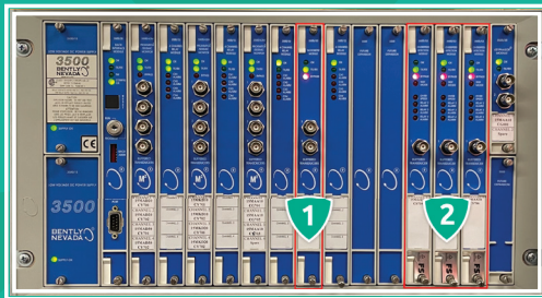
Figure 4 The Bently Nevada 3500 system at AVR. The tachometer module (1) for zero speed monitoring and the three overspeed modules (2) were replaced with the SpeedSys 200. The other cards remain in use.
