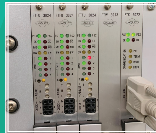
Figure 2 The obsolete FT3000 system configuration that needed a replacement solution.
