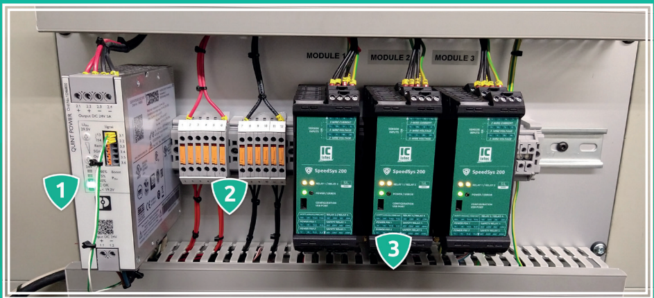
Figure 3 - The new ODS installation consisting of a galvanically isolated SELV power supply (1), a double 24V supply distribution for a possibility of redundancy (2), and three SpeedSys 200 units, hardwired to form a 2oo3 voting structure (3).
